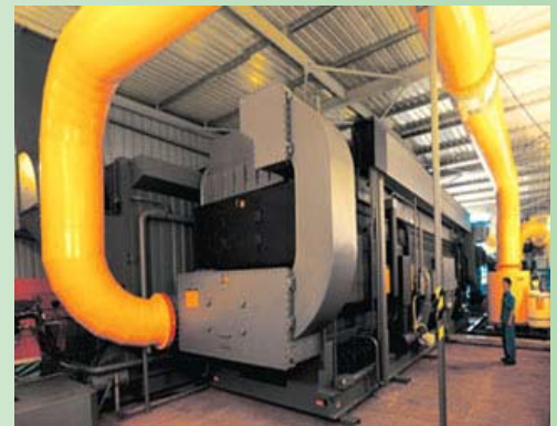
Interior of the BY1000 machine room
